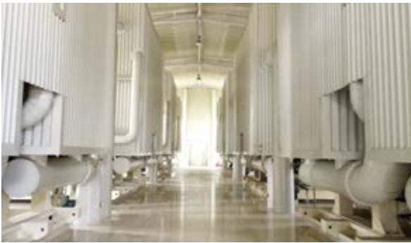
热泵房内部 Inside of heat pump house (view of heat pump unit)
