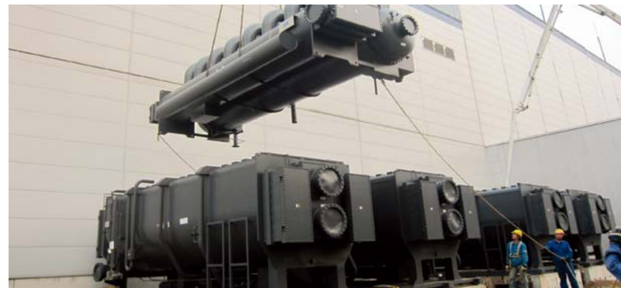
吸收式热泵安装现场 Absorption heat pump assembling in location
