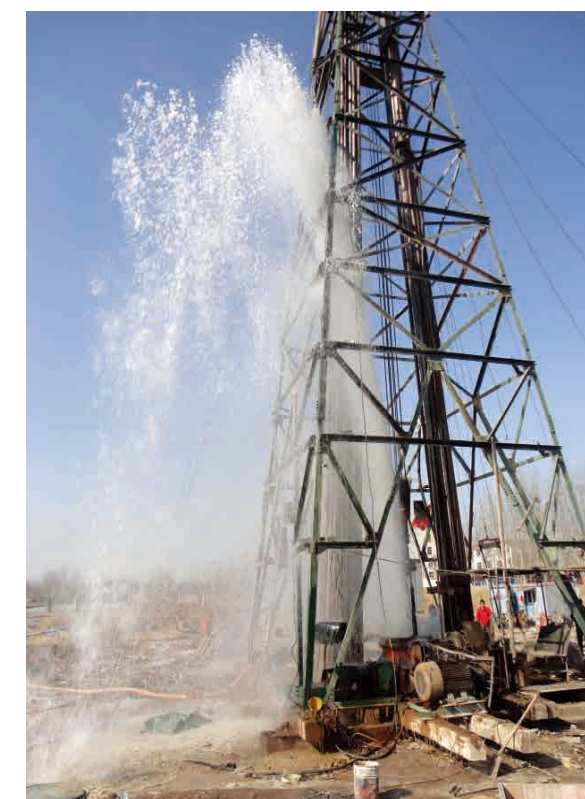
莒县店子集地热井 Ziji Geothermal Well
