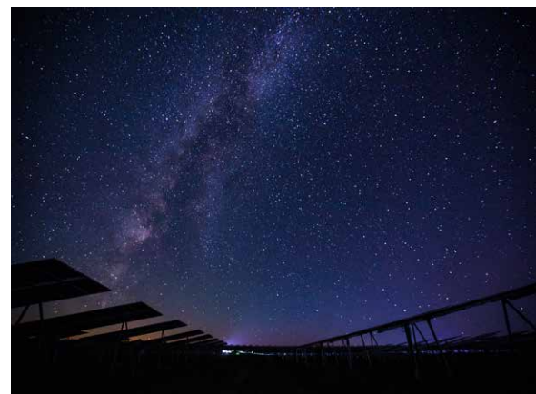
▲ 隆基股份建设的库布其沙漠光伏电站夜景 Night view of Kubuqi Desert photovoltaic power station built by LONGi
