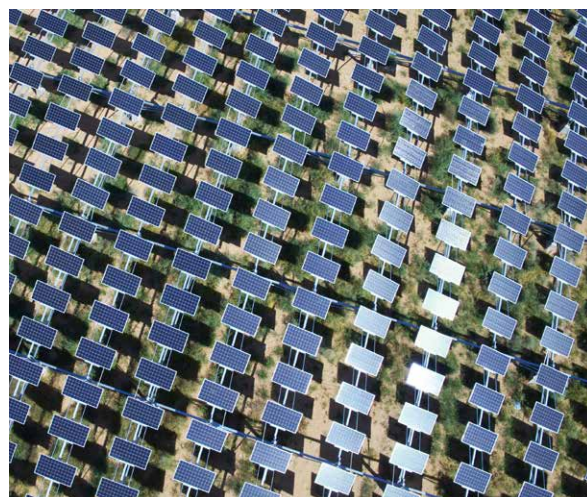
▲ 隆基股份建设的宁夏宝丰集团光伏电站 Ningxia Baofeng Group photovoltaic power station built by LONGi
