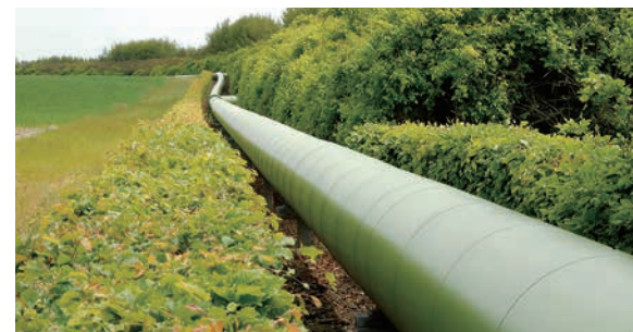
▲ 通向诺和诺德公司的蒸汽 Steam to Novo Nordisk
